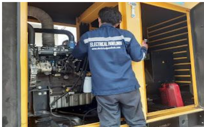
Gambar 2. Maintenance Generator Set
